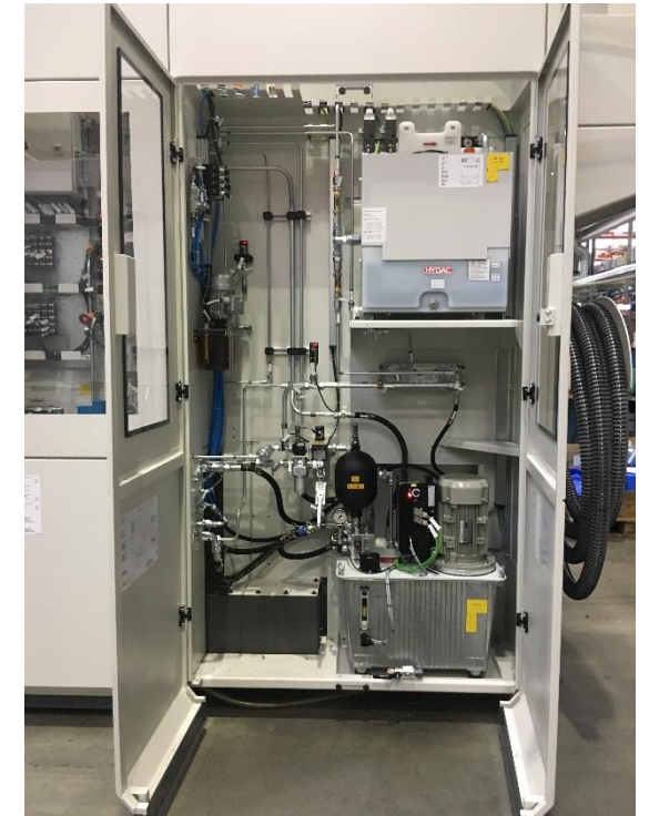
– Opened doors to the hydraulic unit
